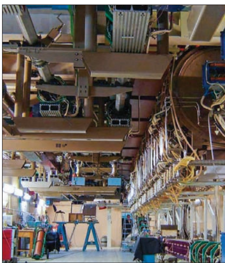
The location of two FELs in the accelerator hall. The original terahertz FEL is at the lower right, with the RF cavities of the ERL above it. Centre left is the new undulator for the bypass FEL.
